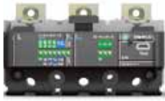
Loose trip units
